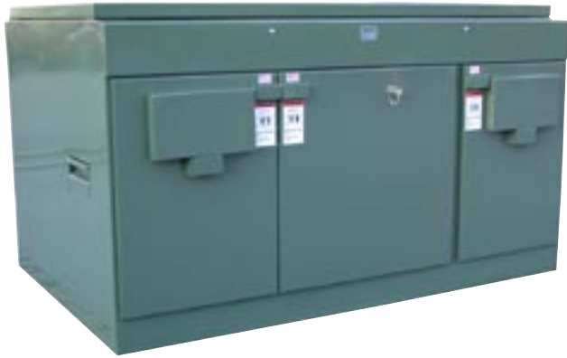
Figure 1a. Exterior view of Primary Metering assembly of FP padmounted switchgear. The compartments on the side pictured above include (from left) incoming switch, metering transformers, and tap switch. Switch compartments include windows on door to allow view of switch position without opening door and security window covers.
