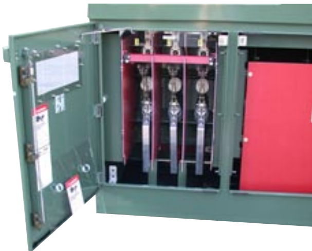
Figure 3. Incoming (line-side) switch with top terminals connected to bus of incoming cable termination compartment and bottom terminals connected by bus to the CTs in adjacent compartment.
