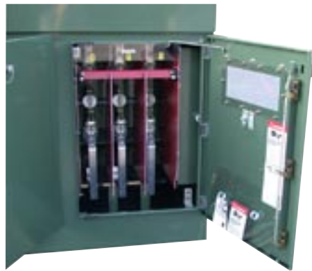
Figure 6. Tap switch pictured here is connected by bus (a) to CTs in compartment on left and (b) to top of fuse terminals in compartment on the opposite side of the switchgear.
